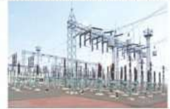
Structure and Transmission Line
